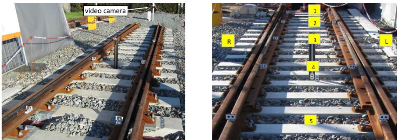
Figure 4 Testing a 1:15 switch panel at Railcenter, Amersfoort. The location 1 – 5 correspond to markers positioned along the switch rail.
