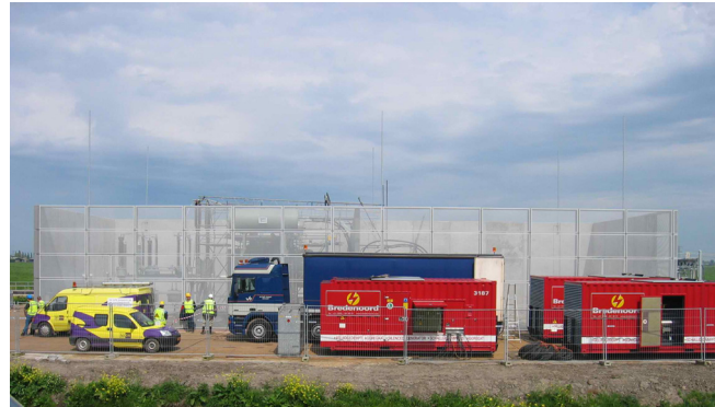
Figure A4: The generator setup
