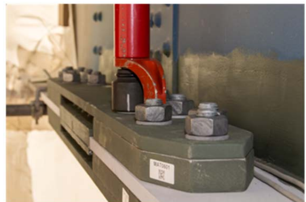
Figure 14. Original riveted connection bridged by a new preloaded bolt connection, Merwede Bridge
